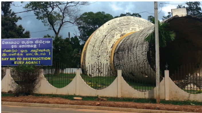
Kilinochchi destroyed water tank
